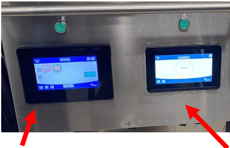
Existing HRCB+ controller (Ultratroniks)
