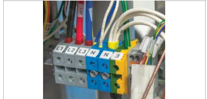
2. WYE Power Supply terminal block.
